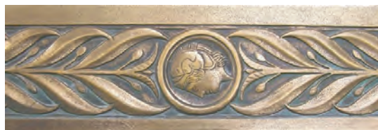
THIS SECTION OF THE ORIGINAL FRAME SHOWS AN EXAMPLE OF THE DETERIORATION. NOTE THE DETAILS ARE WORN OUT, MAKING THE FRAME LOOK FLAT.
